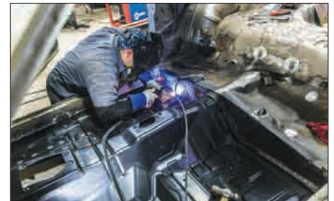
The new floorpan has been seated and clamped to the frame rail extensions and both the fore and aft pans. This full pan is the only way to go if you want solid structural integrity. This way there are no welded seams and the associated weaknesses.
