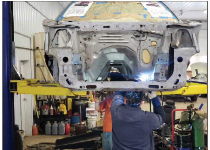
Make sure the body is adequately supported during the structural repair process. If you're doing floorpan, frame rail, or rocker panel replacement, properly support and jig the structure. Everything must be spot on. If it's not, doors, fenders, hoods, and decklids will not line up.
