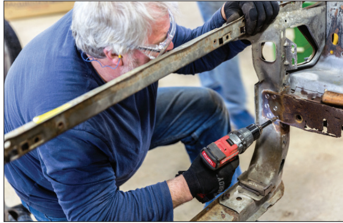
This front frame rail/strut tower assembly suffers rust-through. Spot welds on the inside of the frame rail are being drilled out for removal of the inside skin, which will be replaced and rosette-welded back together.
