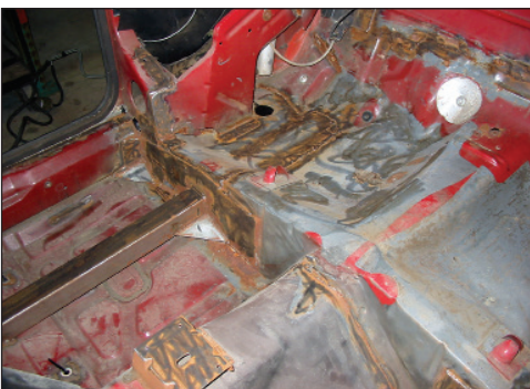
Make sure your patch repairs make structural and aesthetic sense. Although floor repairs typically cannot be seen, they should make structural sense.
